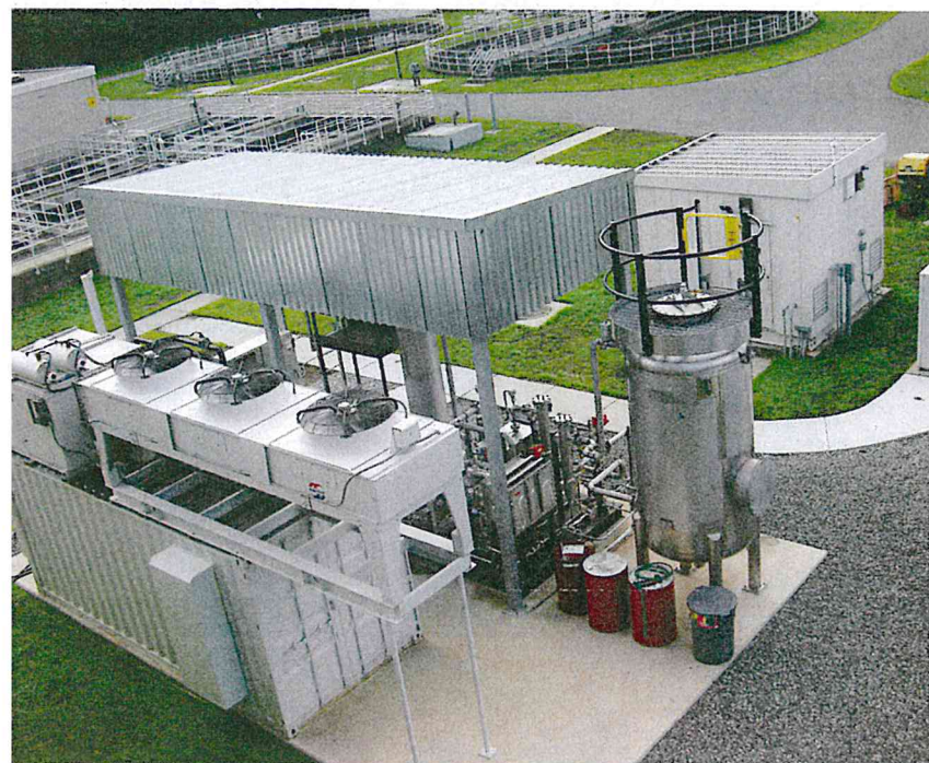
Technology used to convert methane gas to electricity includes anaerobic digesters, a 240 kW engine/generator from Kraft Power, and a 50 kW solar field from Advanced Solar.
