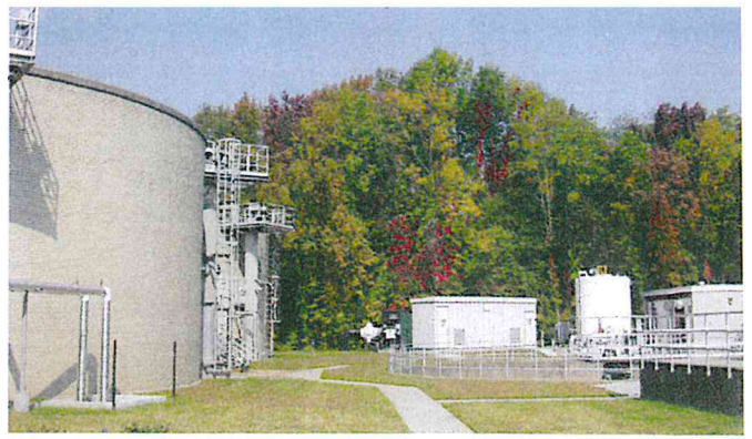
Electricity production is enhanced when food wastes such as fats, oils and grease are added to the process by way of this liquid waste receiving station.
